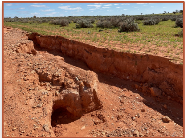
Track erosion due to March rainfall in the GVD. Photo: Pila Nguru Aboriginal Corporation
