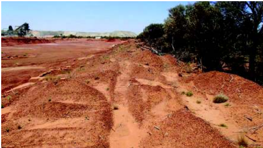
Figure 16. Western End of Borrow Pit Requires Reworking/Filling to Achieve 15 Degree Slope
