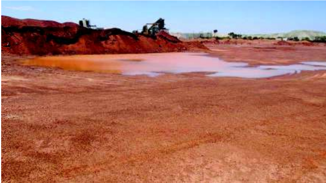
Figure 13. Depression Requiring Fill
