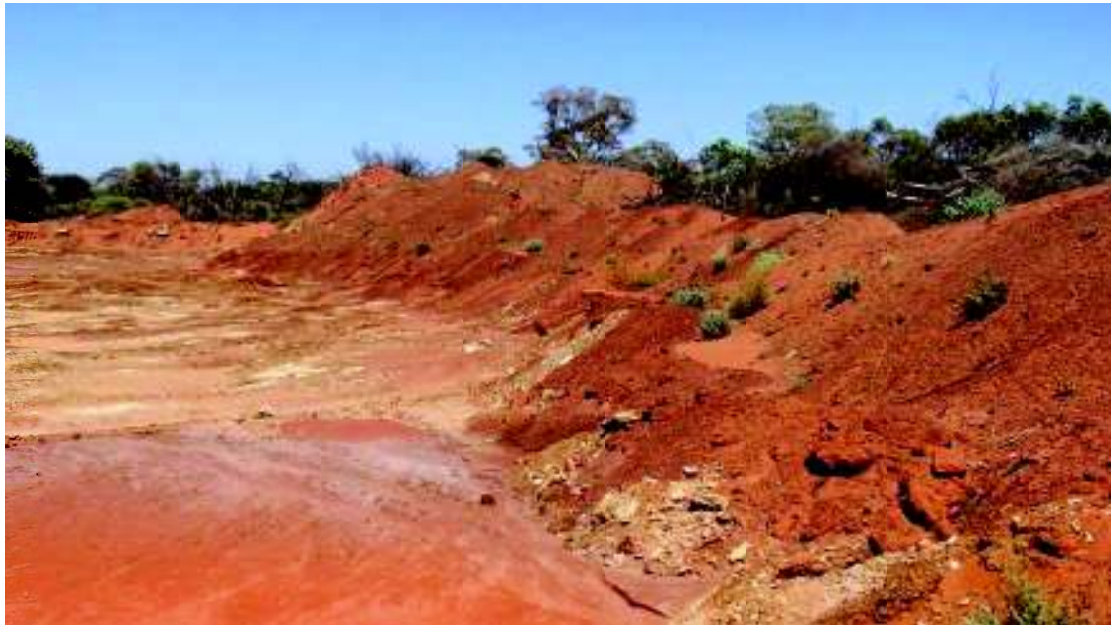
Figure 15. Northern End of Borrow Pit Requires Reworking/Filling to Achieve 15 Degree Slope
