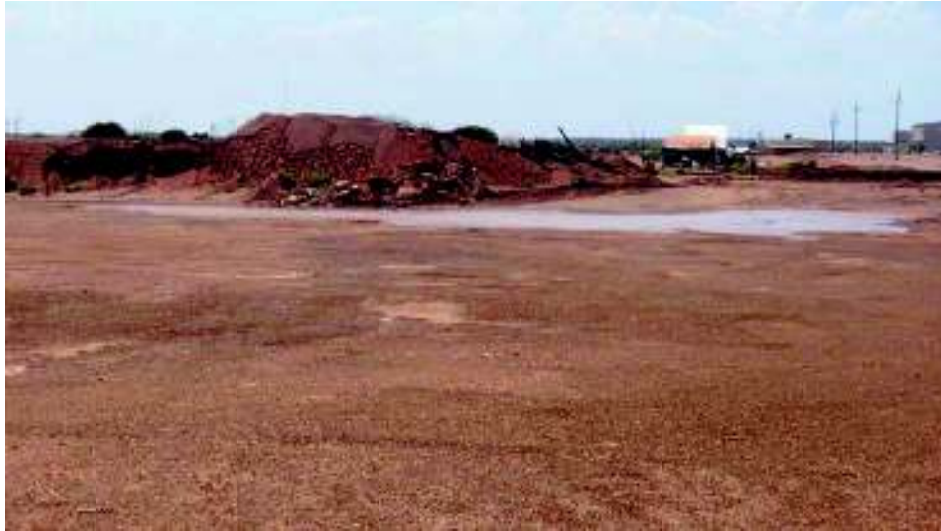
Figure 4. Depression Requiring Fill
