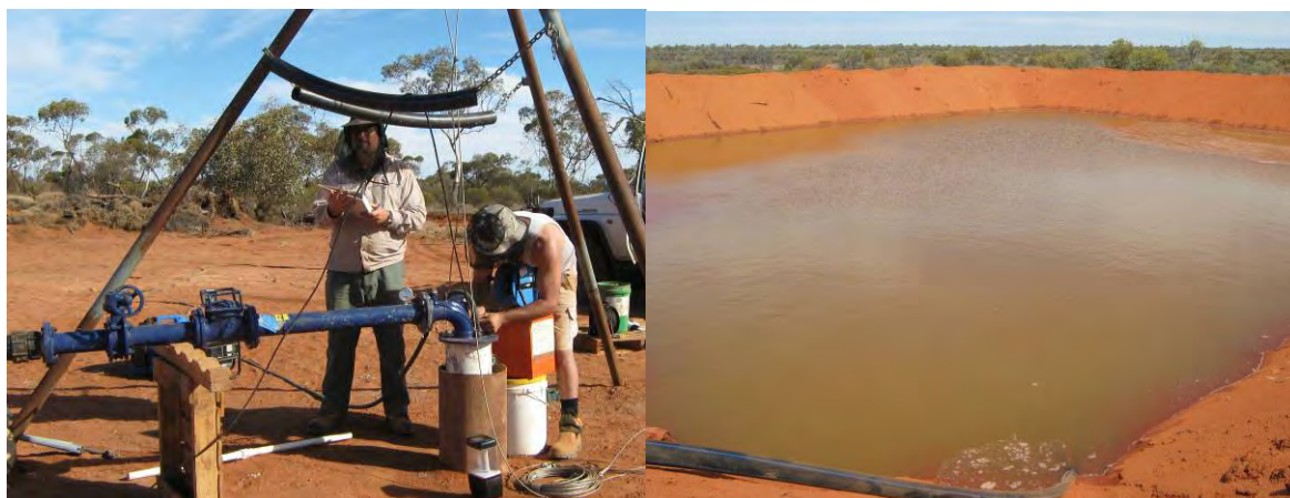
Figure 3-6: Constant rate test pump test being conducted on a test production bore in the Water Supply Area with the saline discharge water captured in a turkey's nest.
